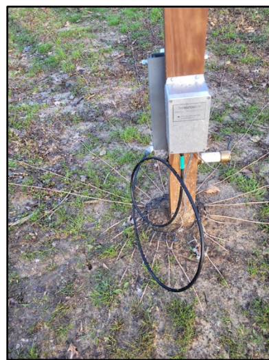
At the Antenna Base: THEMATCHBOX Matching Transformer and Costa's Home-Built Groundplane
