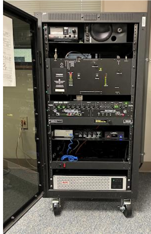
Redmond WA's system above includes Network Audio Management & streaming equipment.
