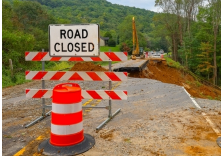
Storm-damaged roads hamper recovery after Hurricanes Helene & Milton.
